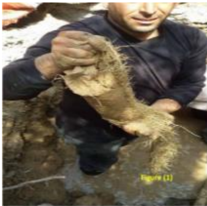
Fig. 1 : shows The roots are pierced in the water pipe in Al-Ressala Sector
