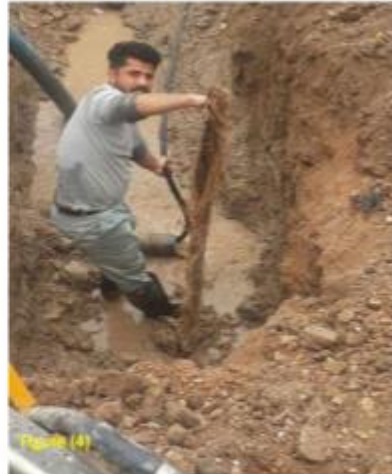
Fig. 4: Shows the roots penetration near to domestic Sewage in Al-Sadekh Sector.
