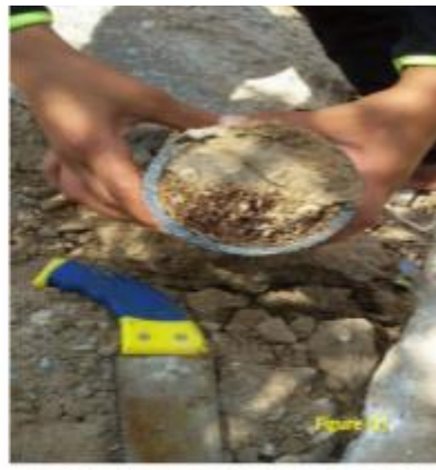
Fig. 2 : Shows the roots penetrated into the water pipe. in Al-Wahla
